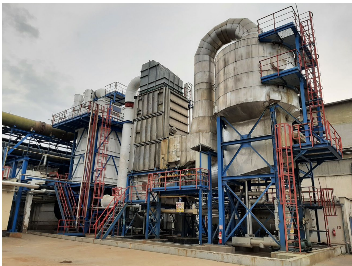
Fig. 5 SULFOX catalytic oxidation unit
